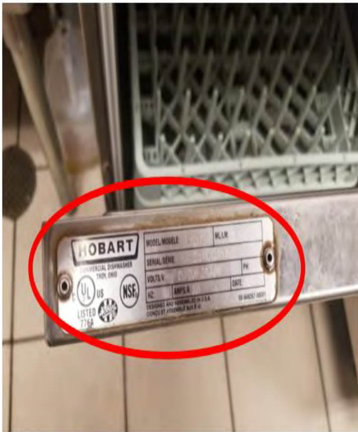
Manufacturer's Plate Location
